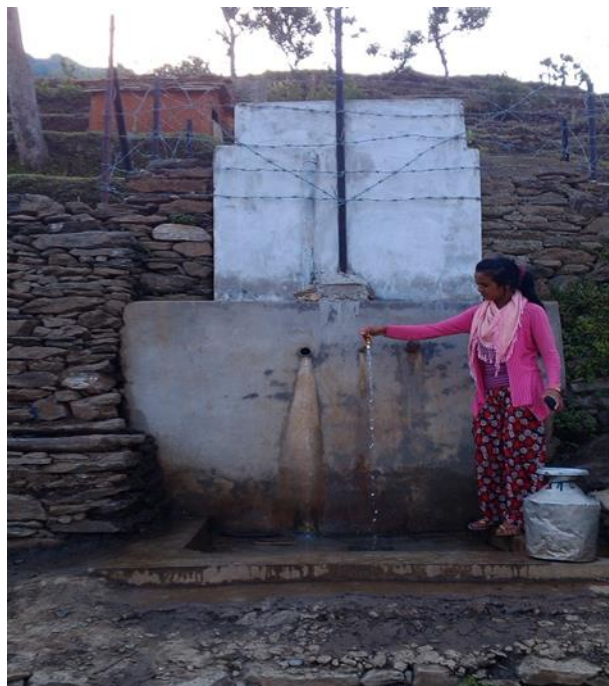
Storage tank with attached Tap
