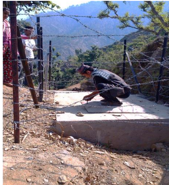
Distribution chamber before storage tank 1
