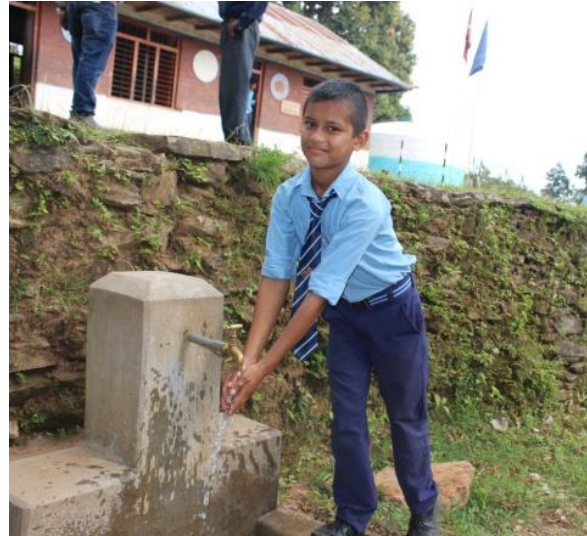
Picture 6 Water point feed from 20m3 RWH tank in Indrayani School
