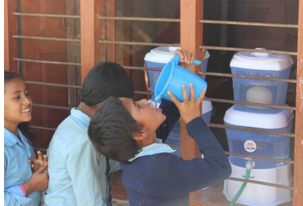
Picture 45 Boys drinking water from newly installed filter in school
